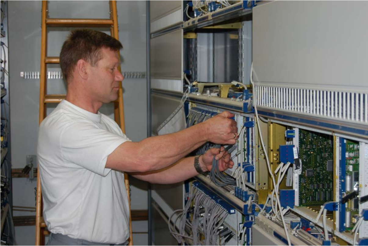
Disconnect existing cabling in the LSM magazine.
